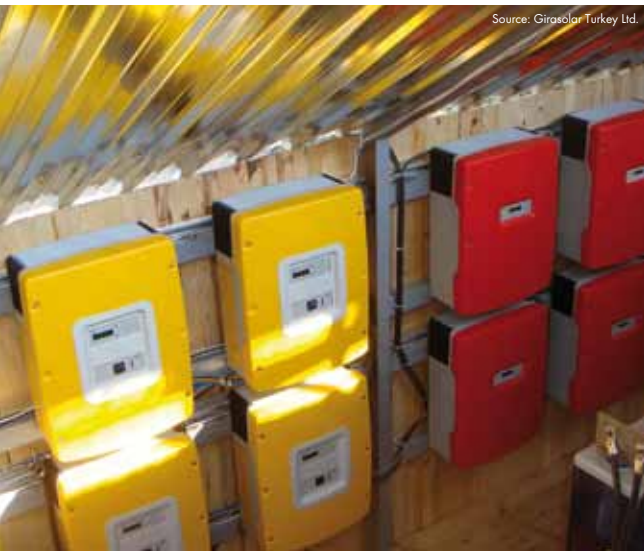
Multicuster-Box 6: Multicuster-Box 6 supplies a restaurant, water purification plant and a cell network relay station with electricity in Kizilada in the Gulf of Fethiye, Turkey.
