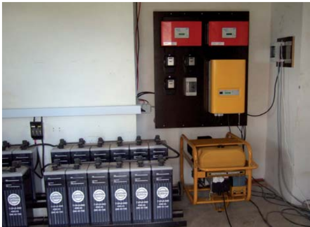
Fig. 9.1: Power supply for a house in Ghana (West Africa)
