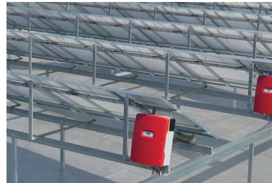
Sufficient electricity for a small city thanks to SMA systems technology Europe's largest solar power plant (as of 2010) in Montalto Di Castro, Italy
