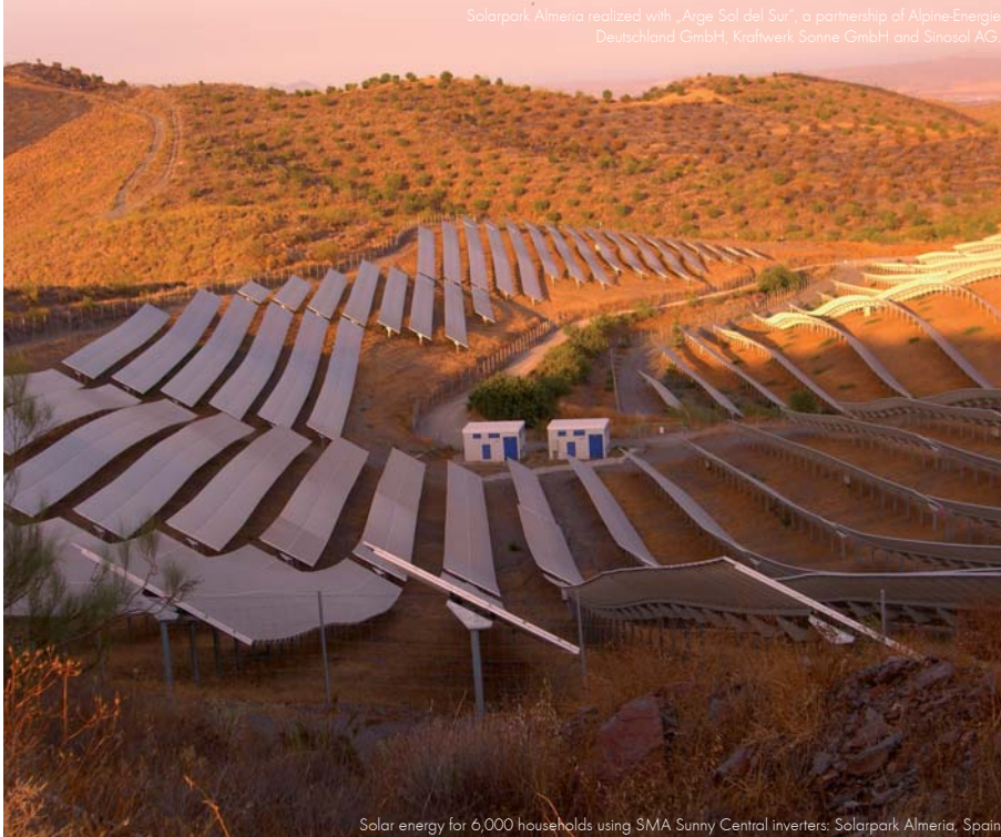
Solar energy for 6,000 households using SMA Sunny Central inverters: Solarpark Almeria, Spain
