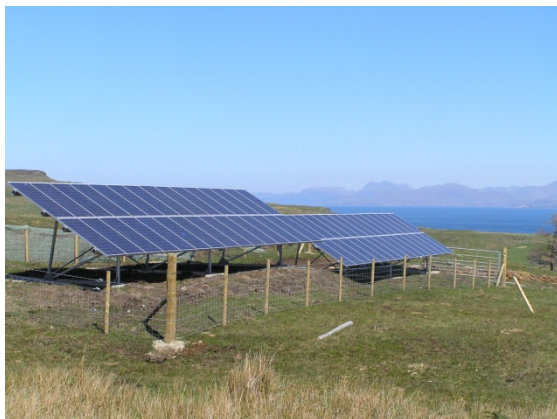
Figure 2: 10 kWp PV array. Additional 22 kWp will be installed in September / October 2010.
