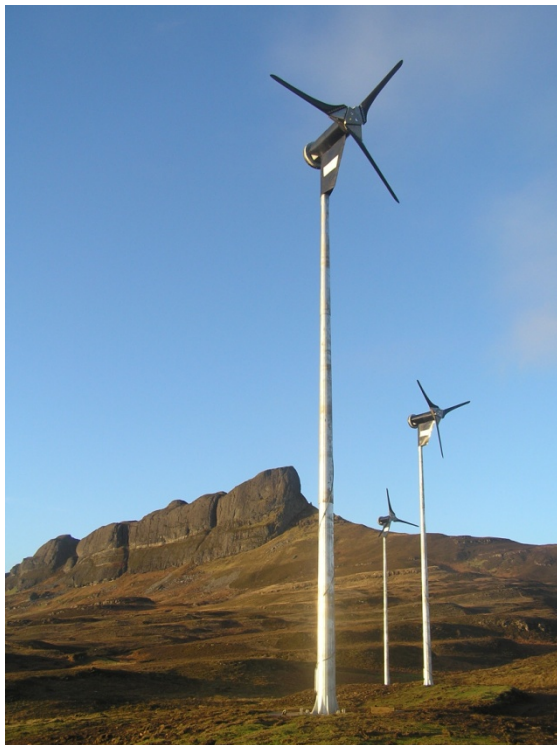
Figure 1: 6 kW Proven wind turbines located in the southern part of Eigg.
