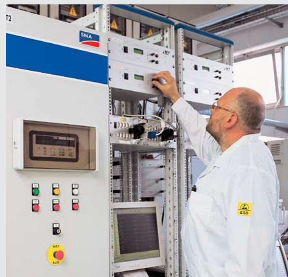
SMA Test Center
